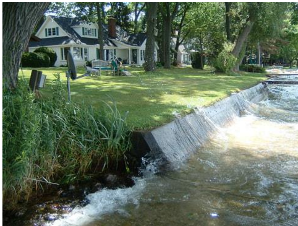
Image 5-6: Example of flanking damage to adjacent shorelines (Photo source: Michigan Natural Shorelines Partnership)
