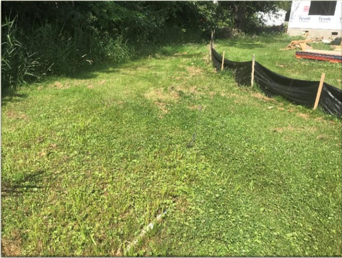
Photo #5: Construction area on the same property from photo 4. There is a dewatering pipe set up to dewater the construction site without the constraint of the silt fence. The intention of the silt fence is to collect sediment before it enters the lake. This drainage prevents that from occurring.
