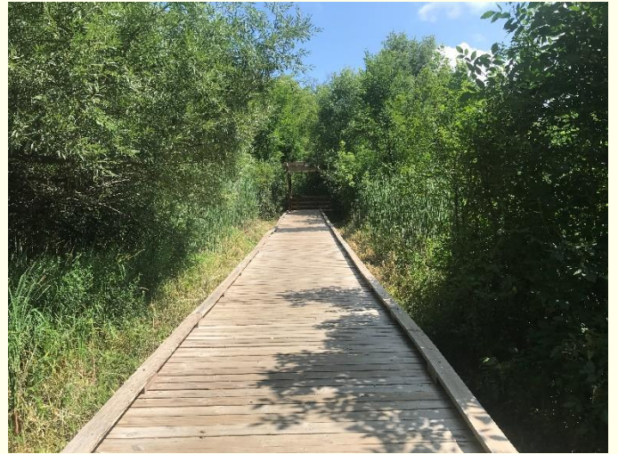
Photo #12: Investments have been made into this property to build and maintain this structure, however the vegetation has been unmanaged, and blocks a view of the lake. This offers little ecological or aesthetic value.
