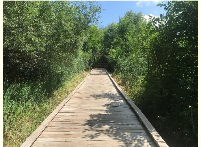
Photo #14: Investments have been made into this property to build and maintain this structure; however the vegetation has been unmanaged, and blocks a view of the lake. This offers little ecological or aesthetic value.
