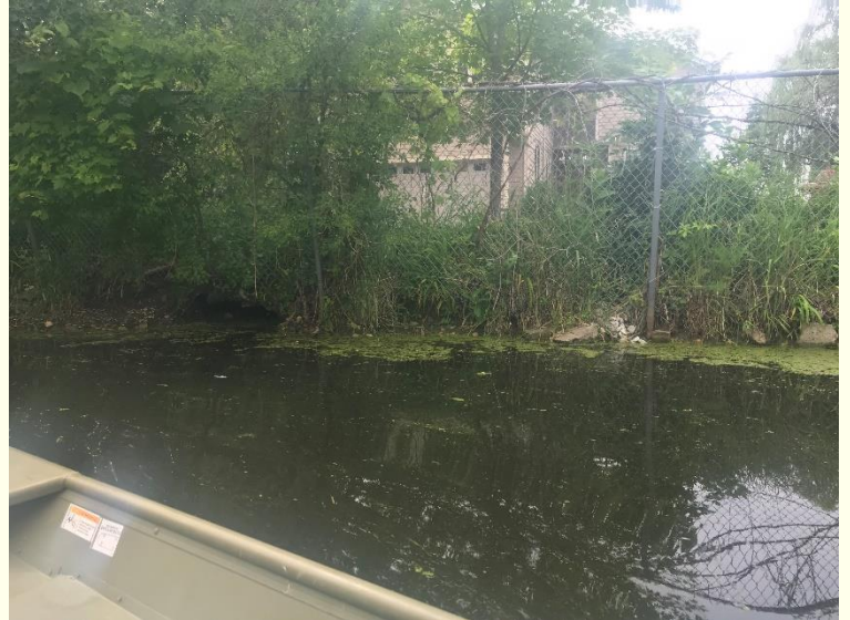
Photo #4: Severe undercutting near the mouth of peninsula channel.
