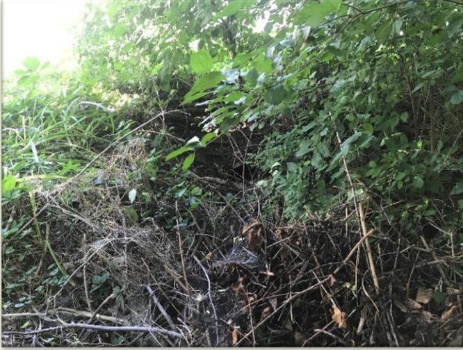
Photo #11: Culvert draining stormwater into the wetland between washington and berger channel.
