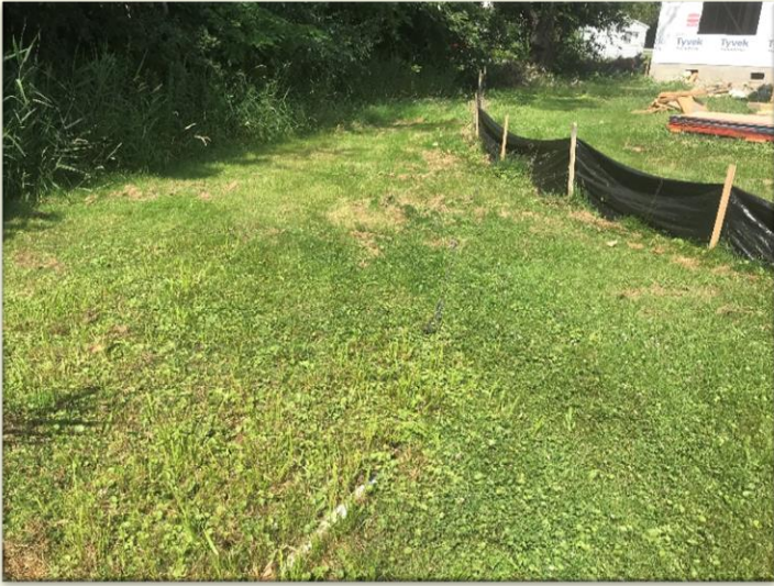
Photo #7: Construction area on the same property from photo 4. There is a dewatering pipe set up to dewater the construction site without the constraint of the silt fence. The intention of the silt fence is to collect sediment before it enters the lake. This drainage prevents that from occurring.
