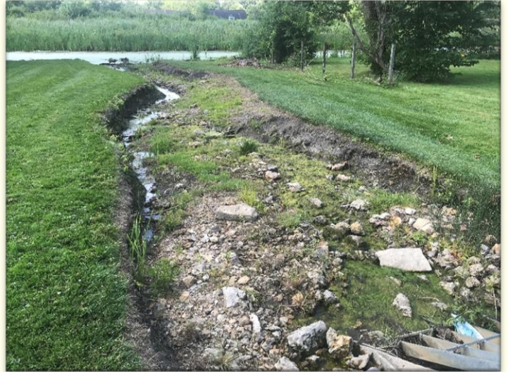
Photo #2: Heavily degraded inlet north of circle channel. Restoration of this area is highly suggested.
