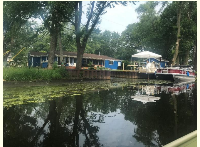
Photo #12: Degrading seawall, unmanaged natural areas.
