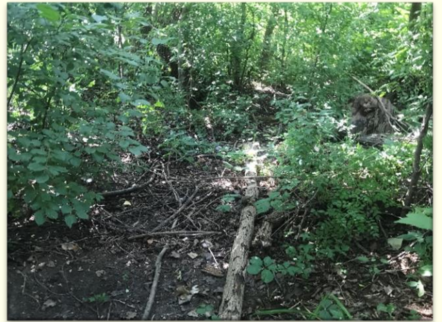
Photo #12: Swale from culvert in photo 9. Overgrown and invaded.
