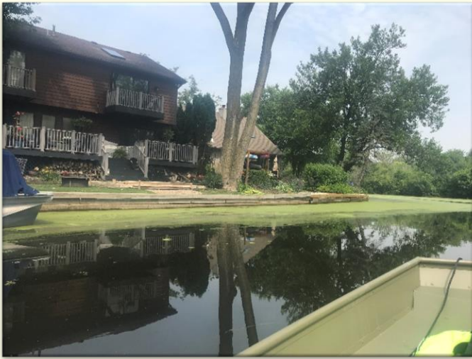
Photo #13: Newly installed timber shoreline control. If maintained routinely, can be effective means of control in areas with limited options.
