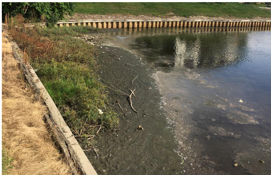
Example of a channel filled with sediment (photo source: ILM Environments)
