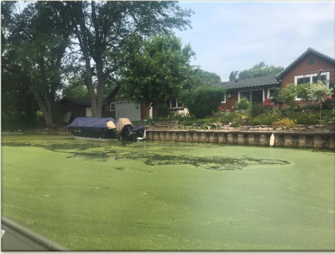
Photo #1: Corroding seawall in circle channel.
