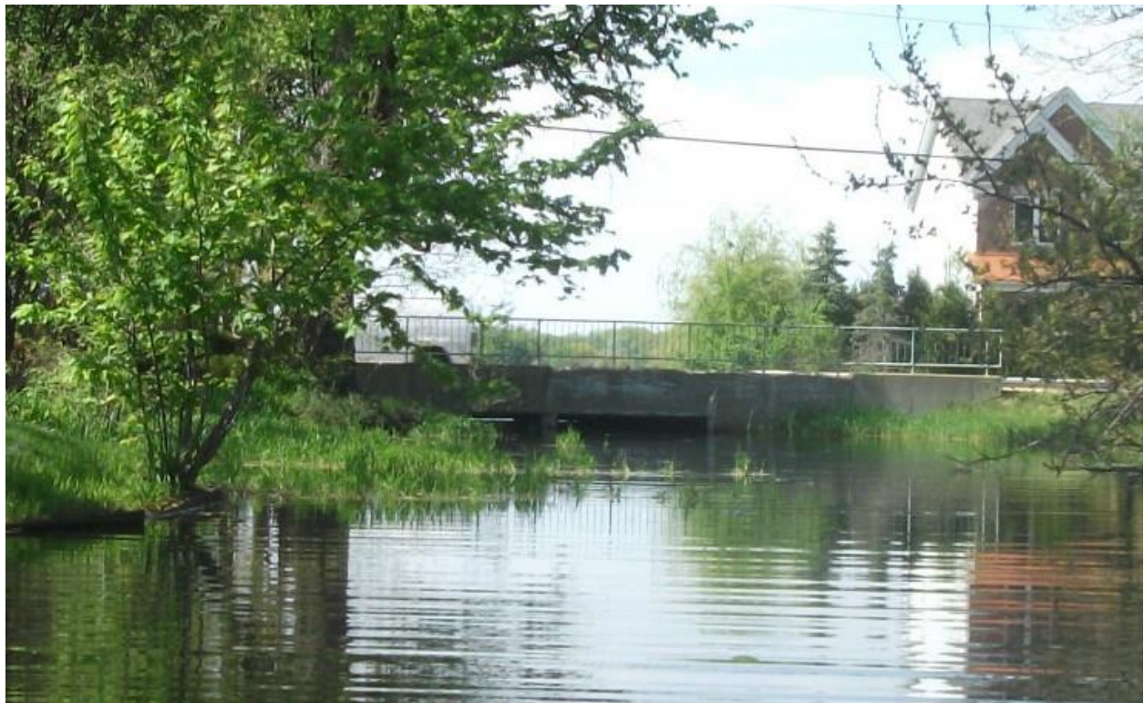
Photo 3-1: Rt. 176 bridge with dam underneath blocking the flow from Kimball Channel to Bangs Lake. Photo is facing north from Kimball Channel.
